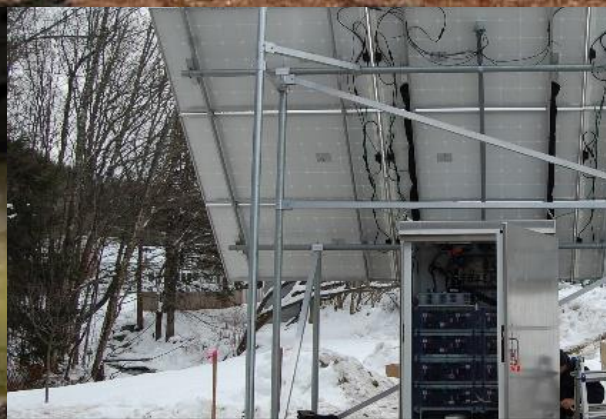
Northern Reliability VTA solar + storage in Rochester
