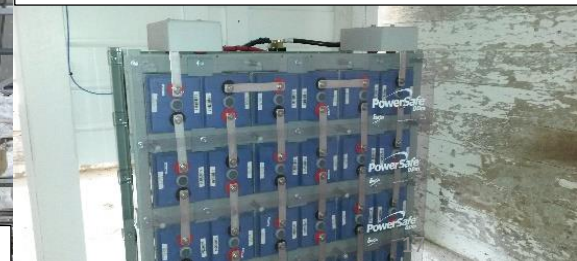
PowerGuru 32 kWh battery in Pownal
