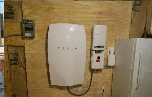
Tesla Powerwall unit installed by Peck Electric in S. Burlington.
