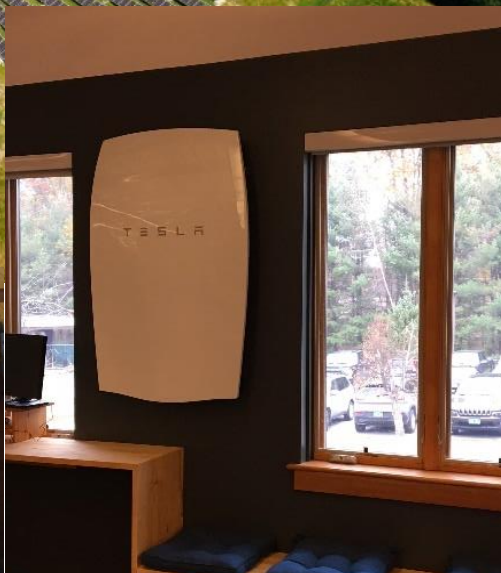
GMP Tesla Powerwall 5.5 kW install
