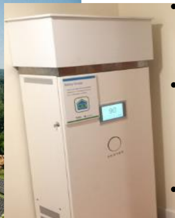
Vermod Sonnenbatteries (6 or 8 kWh) at McKnight Ln. project in Waltham
