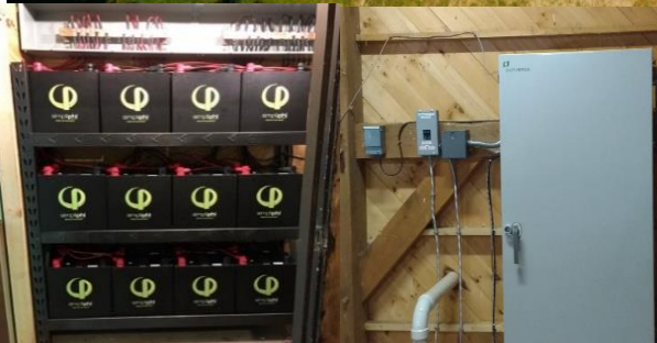
Simpliphi 82 kWh system at Emerald Lake
